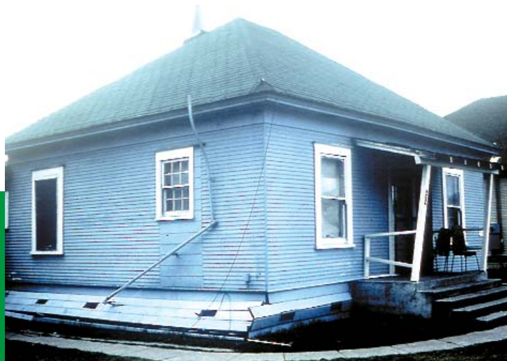
Cripple wall foundation failure, Northridge, Calif.
